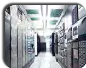
Data Center Management
